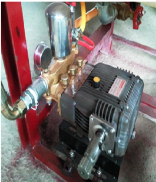
Figure 3. Water pump and main valves
