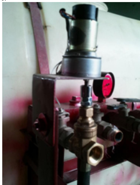
Figure 1. First electric valve
